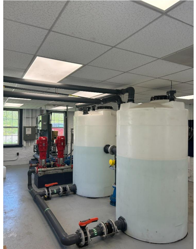
Grindstone Equalization Tanks (prior being pumped into system)
