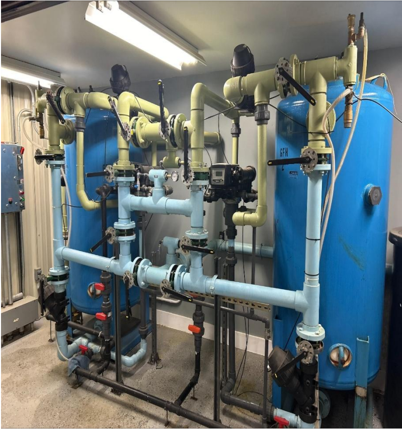
Grindstone Arsenic Removal Media Vessels
